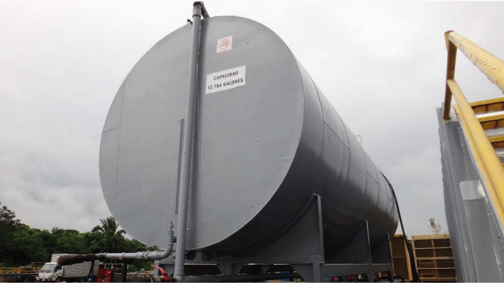
Diesel Tank Cylindrical – Capacity: 10.000 Gal.
